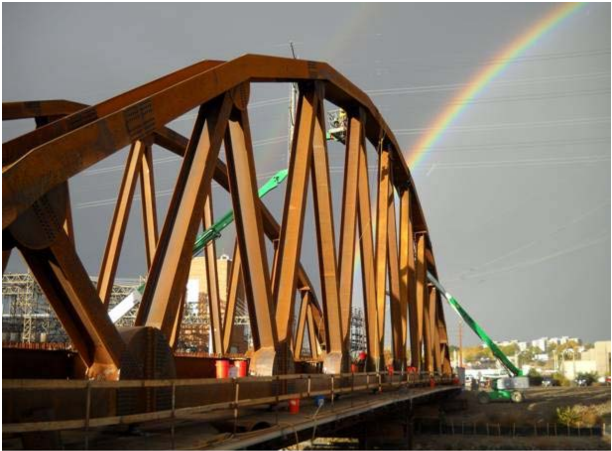
West Corridor light rail bridge construction takes place rain or shine over on the the South Platte River Bridge
