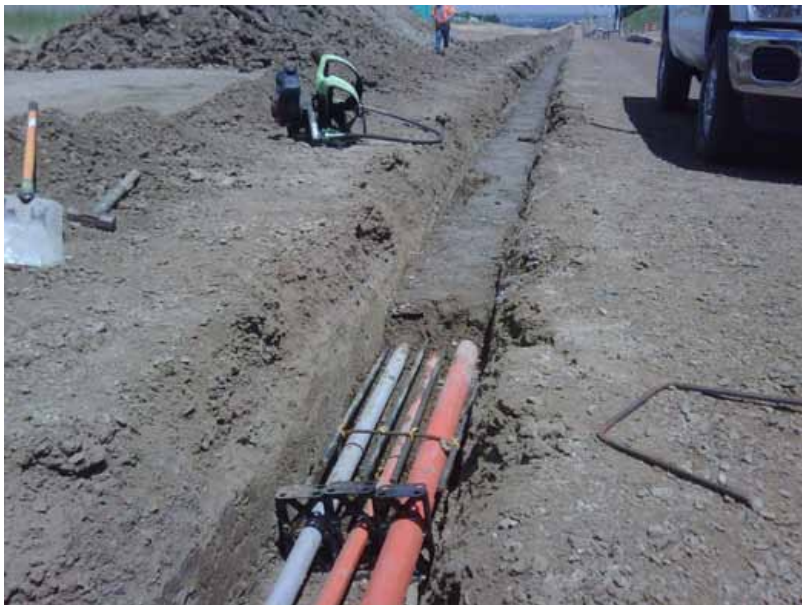
Signal Ductbank Installation Work continued this quarter on the installation of Signal Ductbank along the corridor
