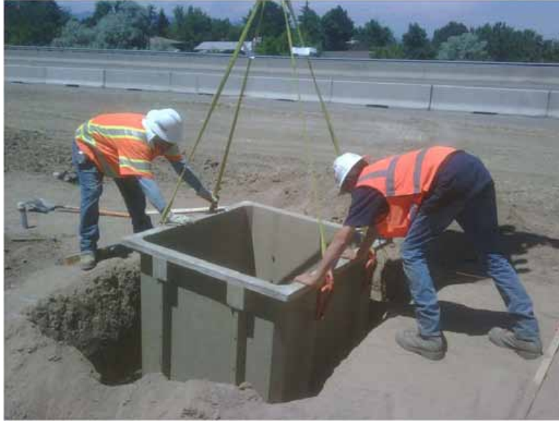
Manhole installation near Red Rocks Station Crews work to install a manhole above.
