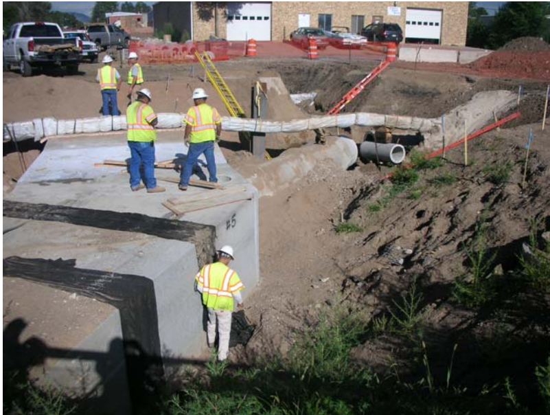
Drainage improvements near Harlan Ct. Crews work on a connection to a drainage improvement being constructed as part of the West Corridor.
