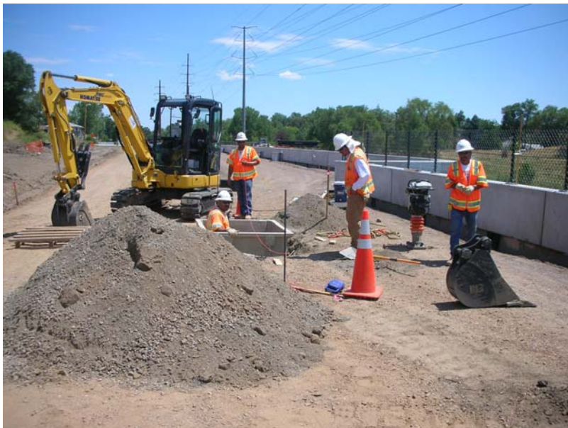
Systems manhole installation Work continued to install facilities necessary for systems that will be installed as part of the project.
