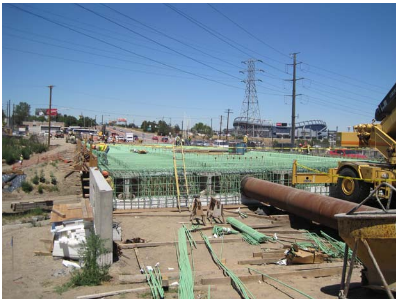
Federal Bridge Work continued on the Federal Bridge, with crews placing re-bar on the structure.
