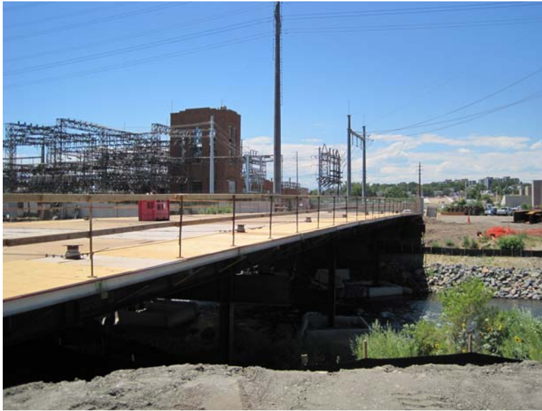
South Platte River Bridge Crews continue to work on the falsework of this structure
