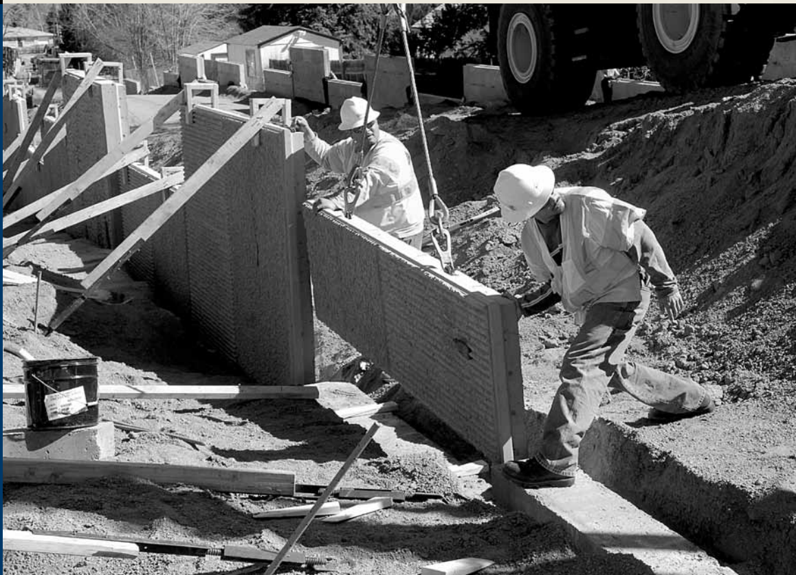
West Corridor construction is in full swing with crews installing retaining walls.
