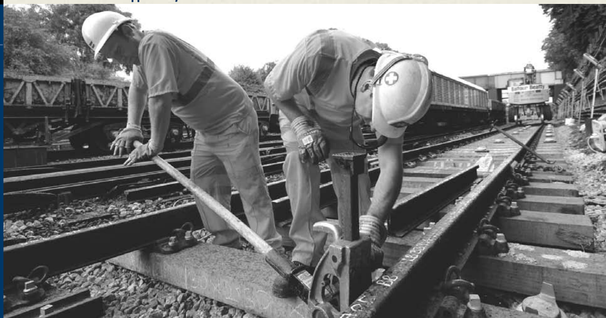
RTD hopes to set an industry model through its mentor/protégé approach to contracting opportunities. Photo provided by Balfour Beatty Rail, Inc.
