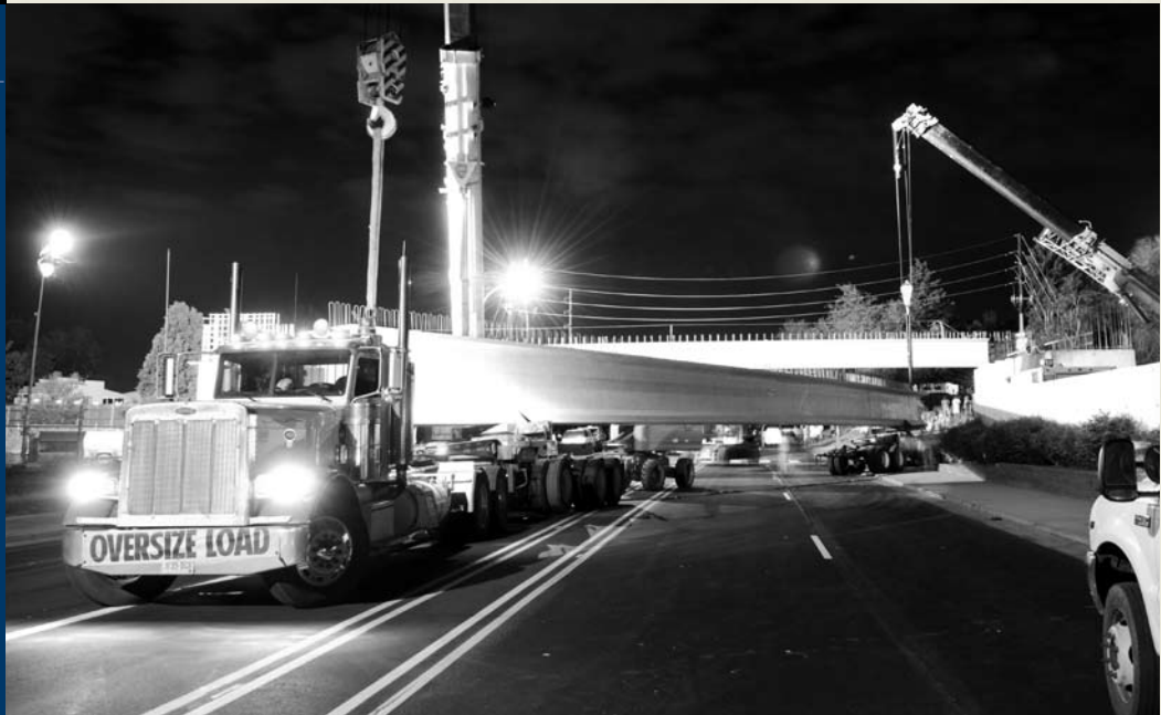
Construction crews erect Kipling Street Bridge at 13th Avenue and Kipling in June.
