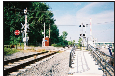
Wayside horn at crossing adjacent to New Jersey Transit Commuter Rail station
