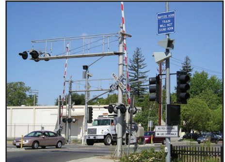
Wayside horn and sign at crossing in Roseville, CA
